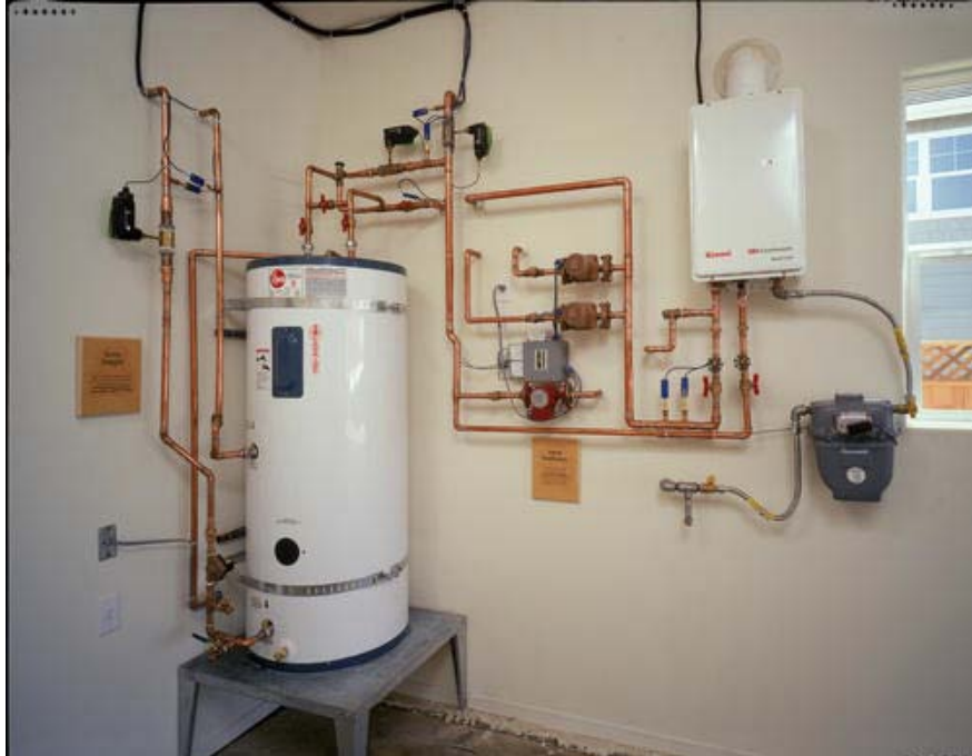
Figure 13. ST system plumbing
